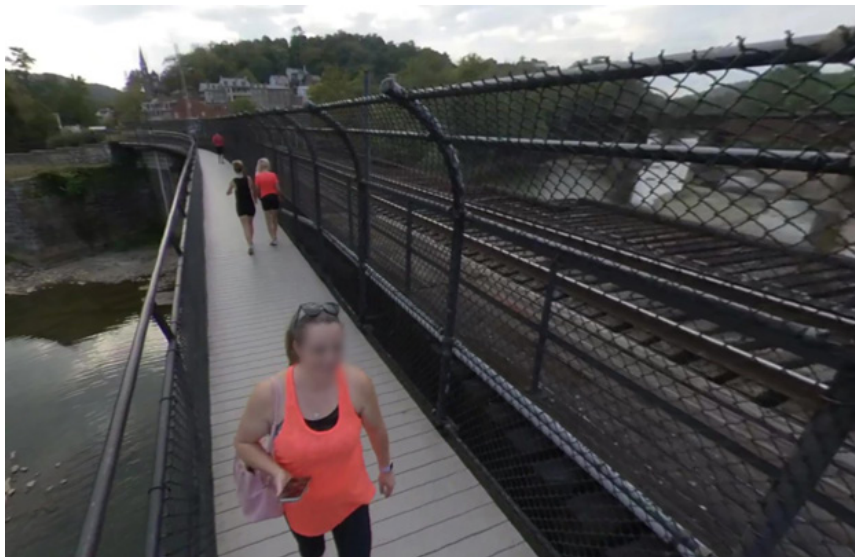
Figure 37 Existing cantilever bridge over the Potomac River along the Appalachian Trail near Harper's Ferry, West Virginia (Source: Google Street View)
